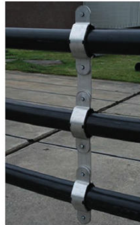
TYPICAL INSTALLATION, PHOTO TAKEN AT A SHORT CIRCUIT TESTING EVENT AT KEMA LAB, ARNHEM NL.
